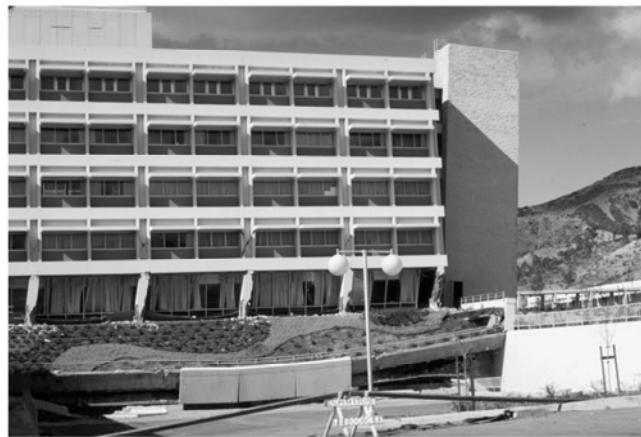
FIGURE 13.5 Permanent offset of weak first story due to discontinued wall, Olive View Hospital, 1971 San Fernando earthquake. (Photograph by K. Steinbrugge, used with permission from the National Information Service for Earthquake Engineering, University of California, Berkeley.)
